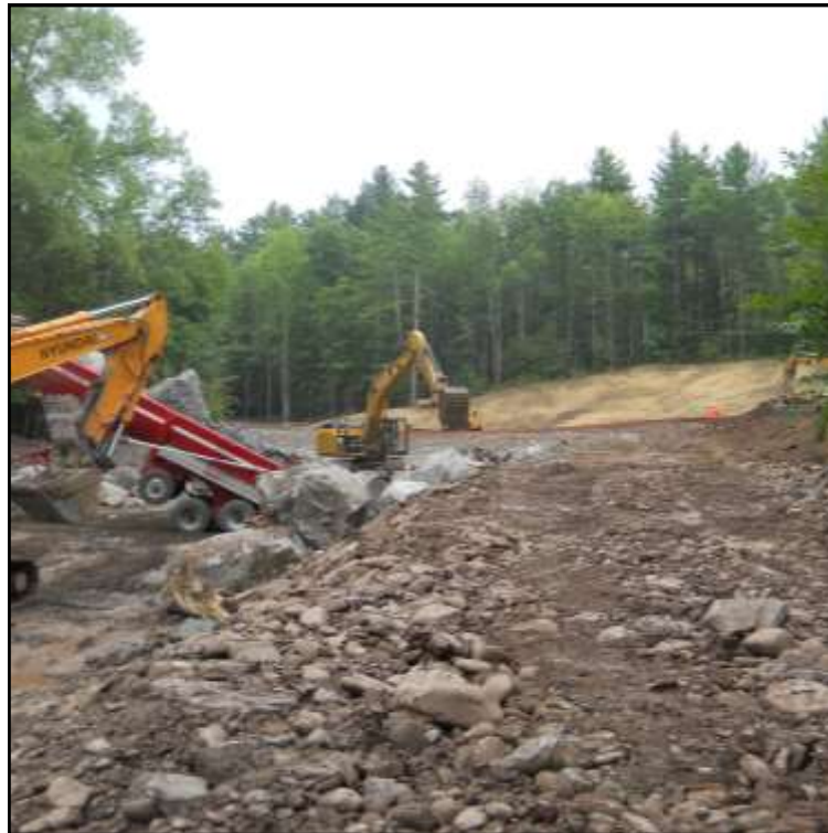
Above: Contractors from Fastracs, Inc. work on a stream restoration project in Chichester, NY during the summer months of 2012.
