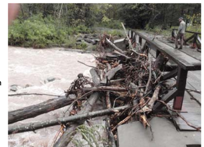
Woody Debris can cause damage to bridges if not removed or there is not enough space for the debris to pass under the bridge
