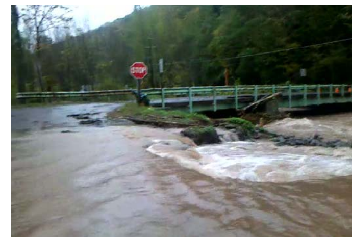
Brown Road in Olivera, damaged by flood water by McKinley Hollow Bridge
