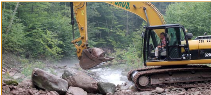
Above: AWSMP oversaw the construction of a stream restoration project on Woodland Creek to stabilize the channel and improve water quality.
