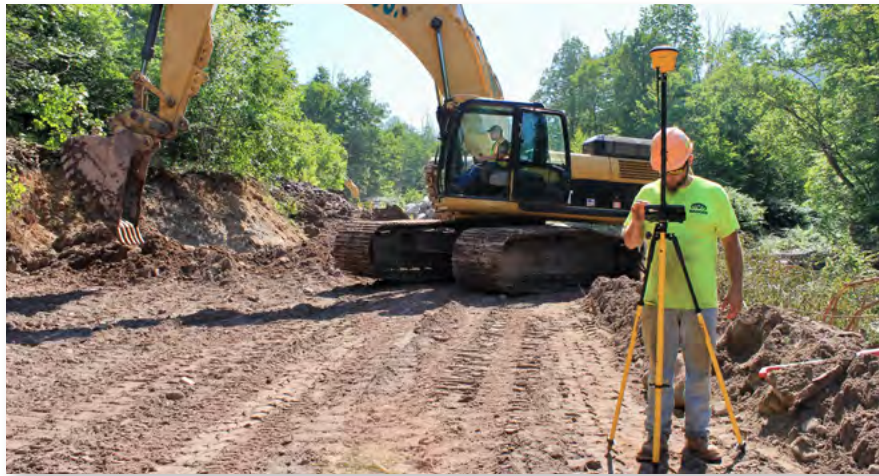
Joe Simorelli of Kingston Equipment Rental & Baker Brothers Excavating uses a survey grade Global Positioning System to mark the future boundary of a stream channel.
