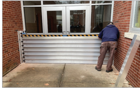
A staff member at Townsend Elementary School in Walton, NY practices installation of a removable flood barrier at one of the building entrances. Photo: CWC.
