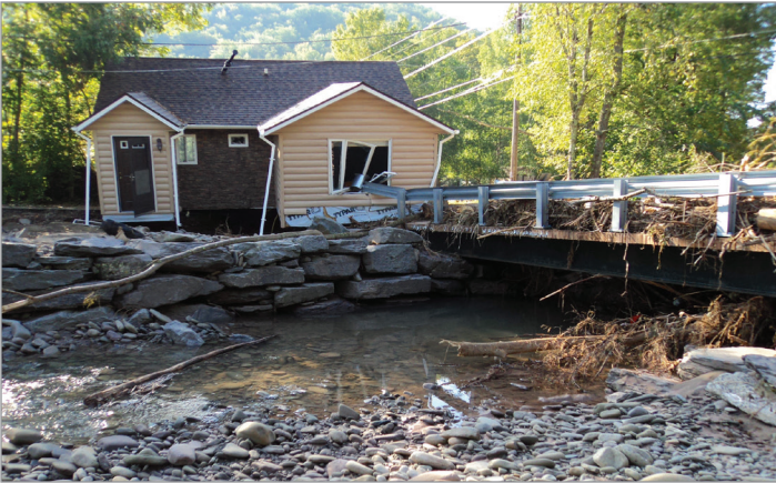
A flooded home pushed off its foundation by floodwaters, Oliverea, NY. This home was not elevated or wet floodproofed. Photo: A Bennett
