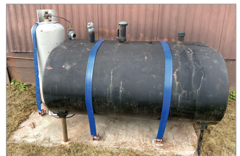
An anchored fuel tank near Halcottsville, NY. Photo: CWC.
