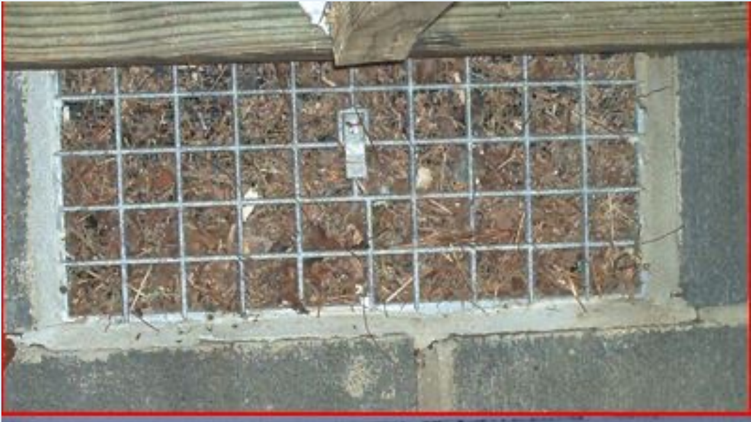
Non-Engineered Flood Vent with Cover that can Trap Debris
