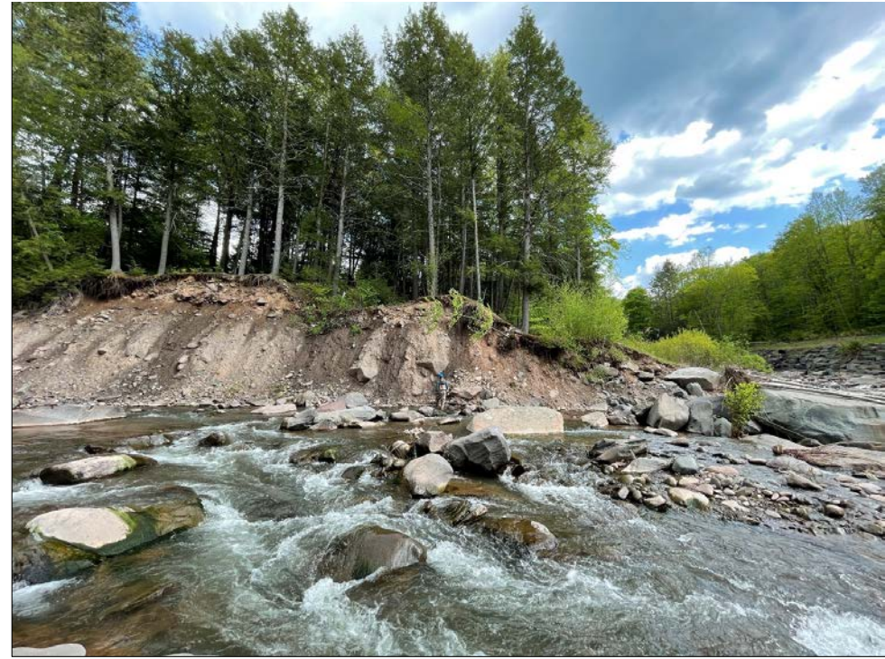
Eroding terraces on Stony Clove Creek, Esopus Creek Watershed
