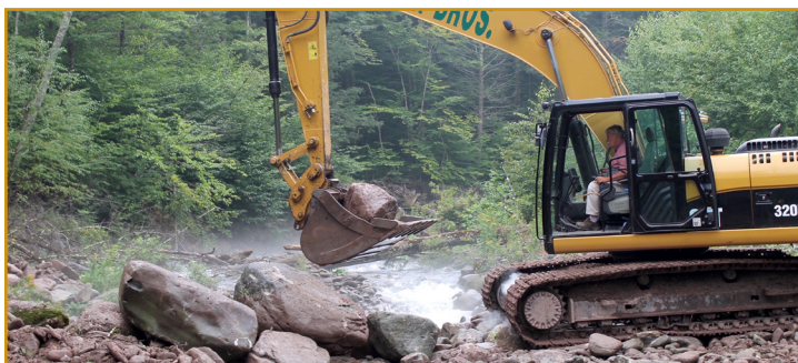
Above: AWSMP oversees construction of stream restoration projects to stabilize and restore stream channels and improve water quality.
