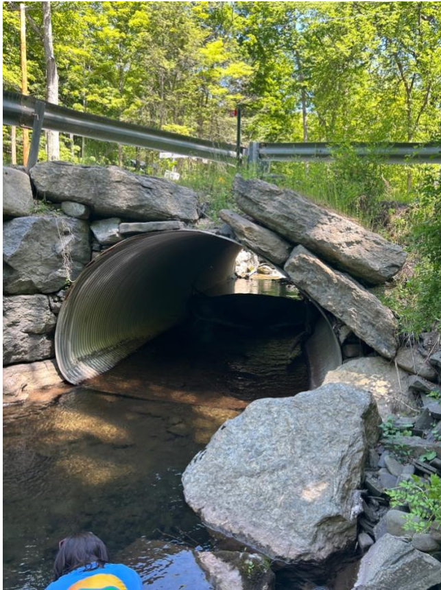
Silver Hollow Road at Lane Road intersection. Failing culvert.
