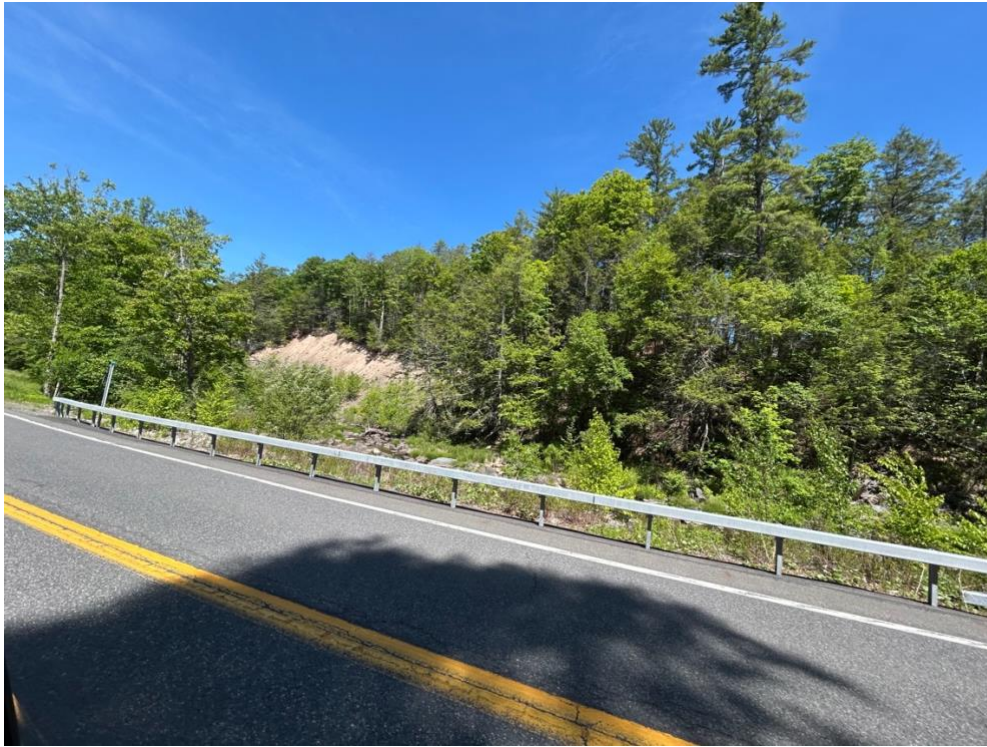
Large failing hillslope (moraine) bordering NY-212.
