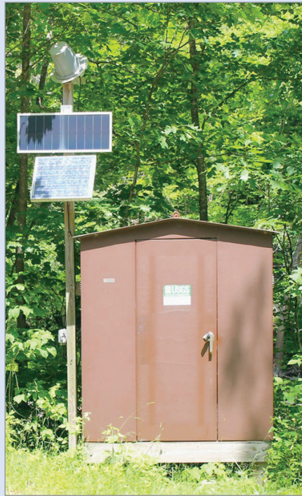
Stream gages are positioned throughout the Ashokan Watershed.
